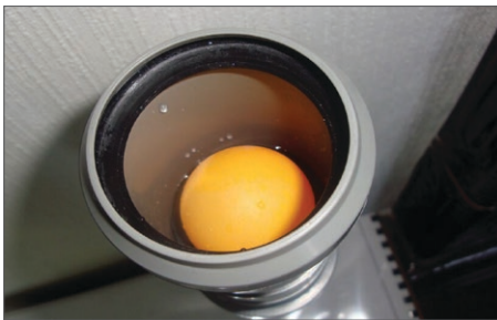
Solution 2: table tennis ball installed below the urinal. Photo from Dima Mamaliga, Apasan, Moldova
