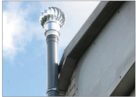
Example of an active ventilation system with wind-driven rotor
