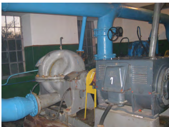
Engine room at the water supplier
