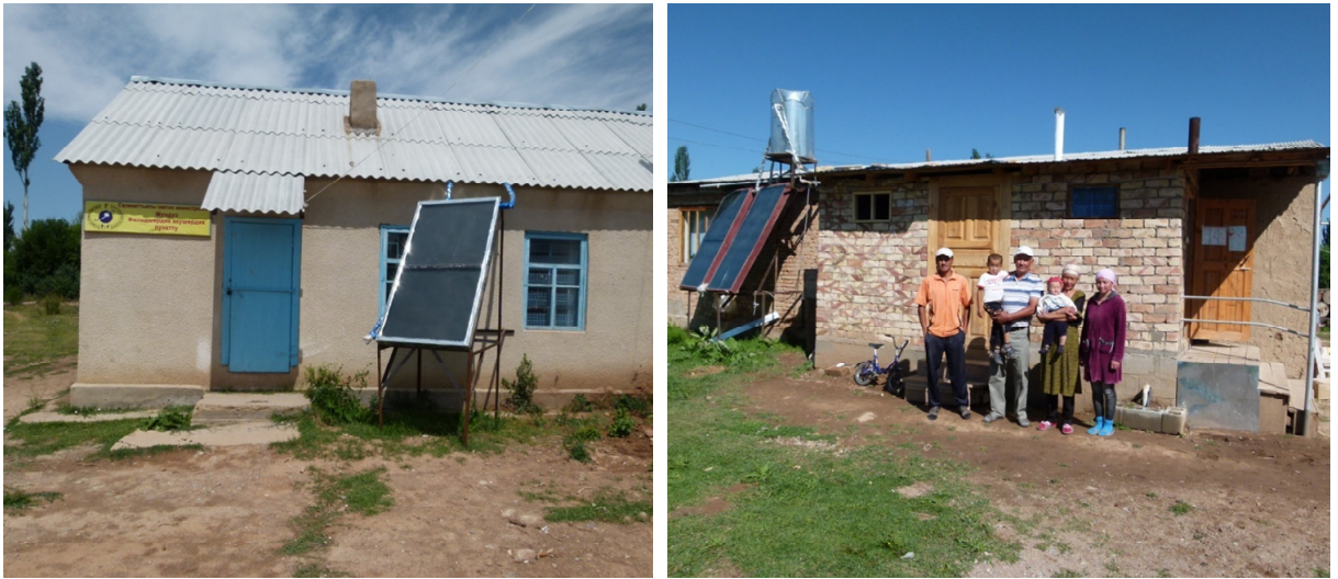
Solar water heater for a school / at the resource centre in combination with a UDDT in Chyrak
