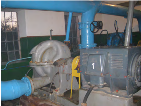
Engine room at the water supplier
