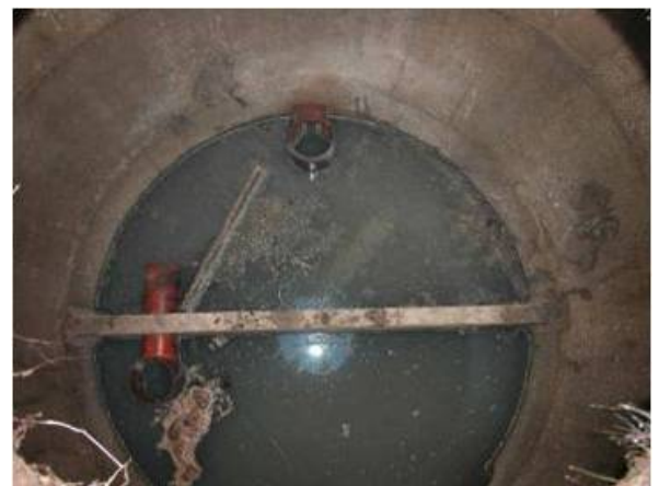
View into the settling tank for pre-treatment of greywater
