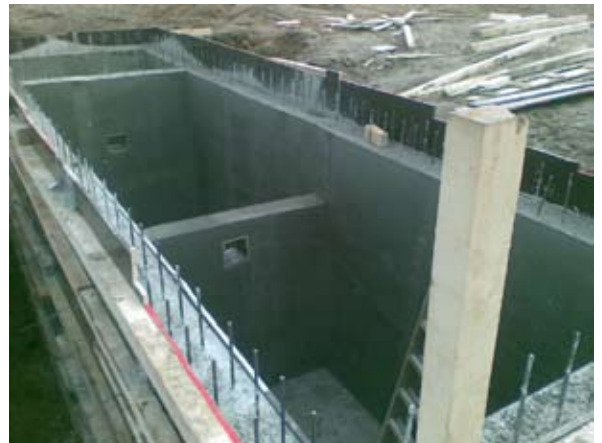
Pre-treatment step: 2 chamber settling tank. 3 rd chamber pumping shaft
