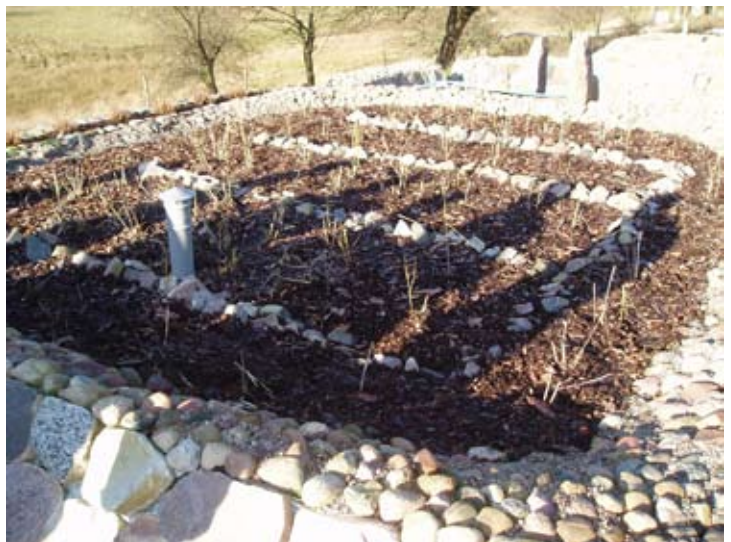
Constructed wetland for domestic wastewater treatment in Poland
