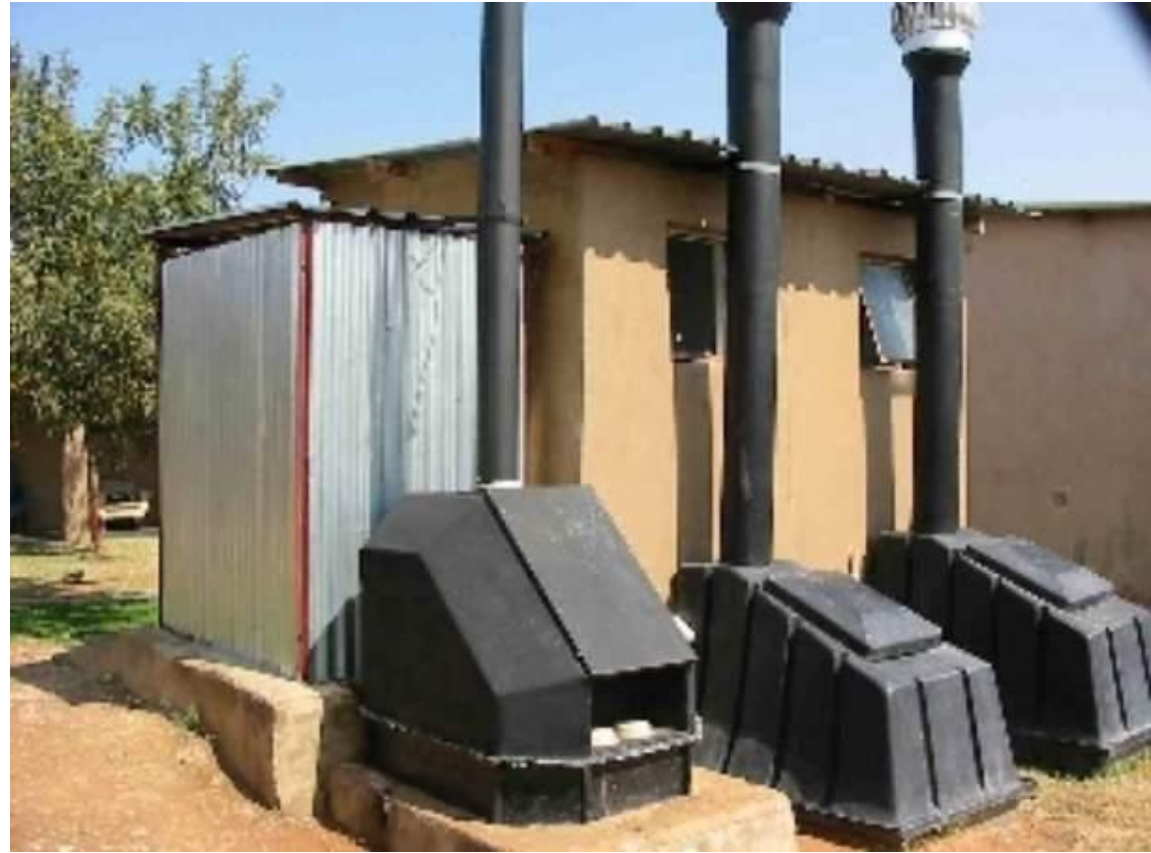
“Enviroloo”-prefabricated system, South Africa
