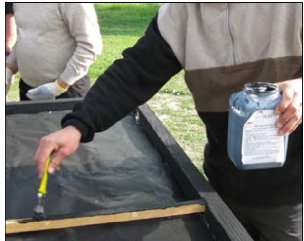
Step 12. Put connection wood bar for glass installation in the middle and cover with black matt paint
