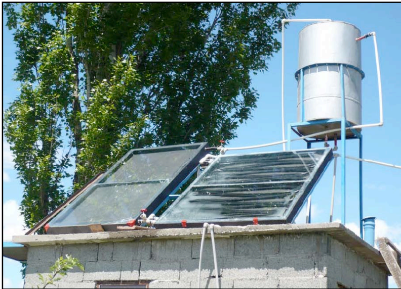
Low-tech Solar Water Heater in Georgia (source: Rostom Gamisonia)
