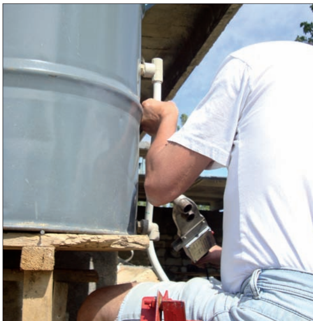
Step 6. Connect to the collector (upside: water in, downside: water out) and to the water supply system (downside: cold water in from storage tank or water supply; upside: warm water out to user)
