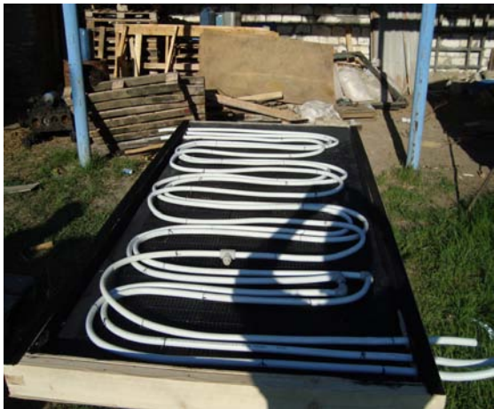
Step 11. Adjust the serpentine pipe to metal mesh in the frame and paint black
